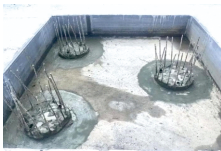
桩头部位渗漏
